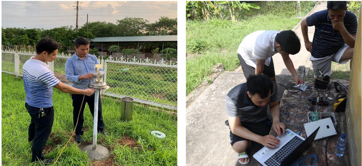
Figure 4.1: Experimental installation of the sensor system at Ha Dong meteorological station and Nhu Tan hydrological station
