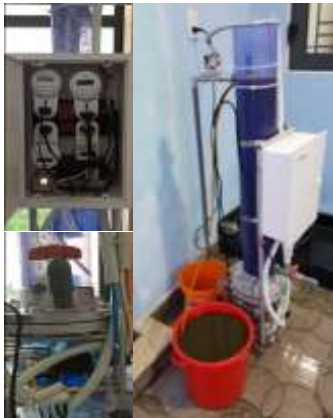
Figure 2.1. Image of SBR system
